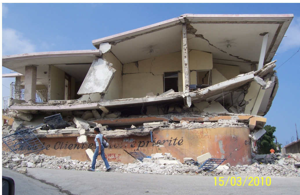
A partially collapsed building in Port au Prince
