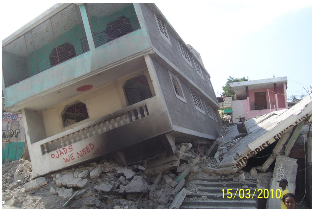
Damaged building showing collapse of the lower storeys
