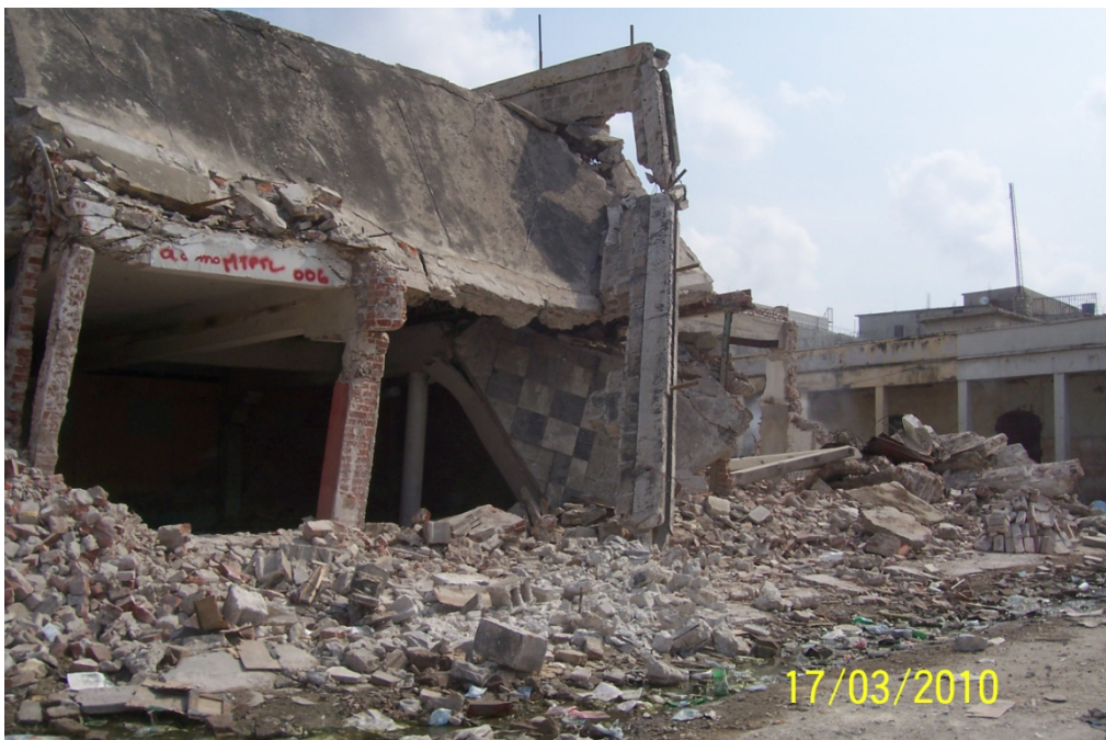
Damaged concrete structure Port au Prince
